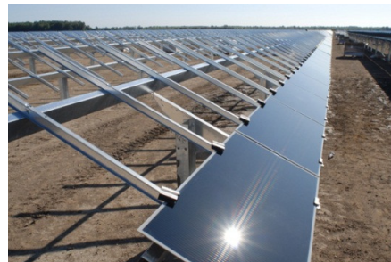
Figure 1: Mounting structure for a utility-scale CdTe PV project.
